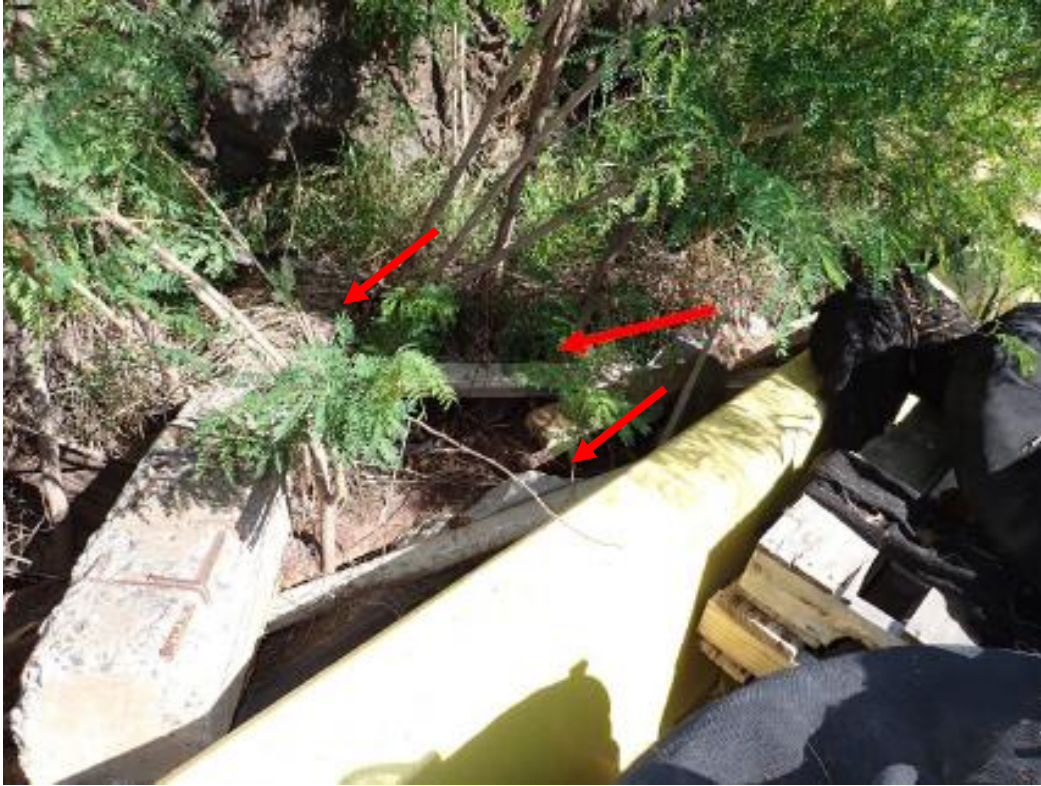
Photo 7: Miscellaneous Items Behind Pile Butt to be Removed
